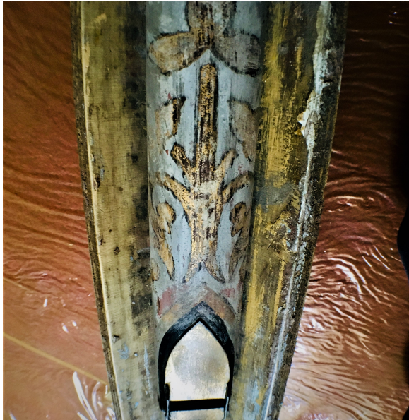
Victorian pipe decoration revealed
