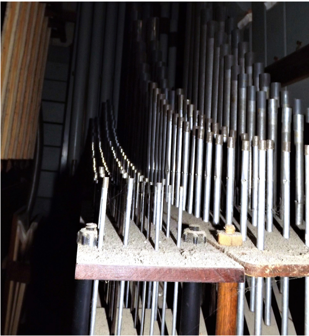
Dust & dirt build-up to Great pipework
