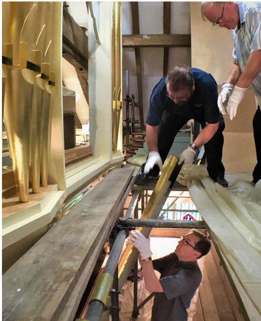
Rector organ builder and organist all lend a hand passing up pipes through the scaffold!
